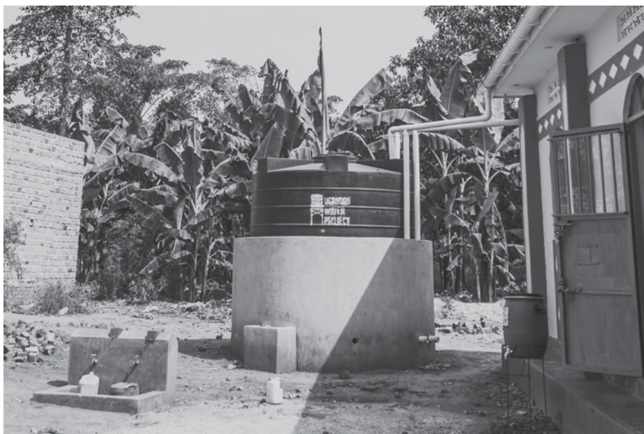
Photo 1 Photograph of a completed RWH system installed by the Ugandan Water Project
